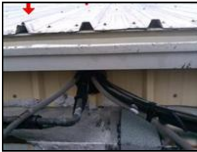
6.0.A Picture 2 Missing closure strips
