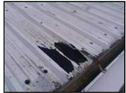
6.0.A Picture 3 Prior repairs noted. Improper material used.
