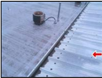
6.0.A Picture 1 Paint worn off
